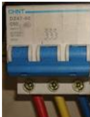
Picture 8 Air Switch
