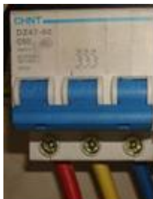
Picture 8 Air Switch
